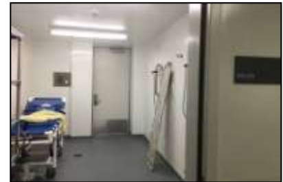
Chemical contain clear room(inside)
